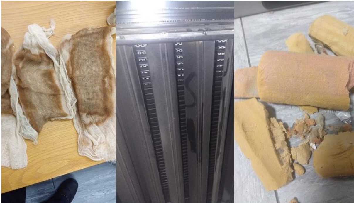
Left: These tack wipes show dust that was found on plastic composite walls, the data hall has Free Air
