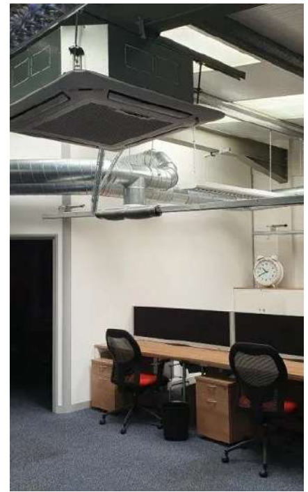
Air conditioning and Ventilation
